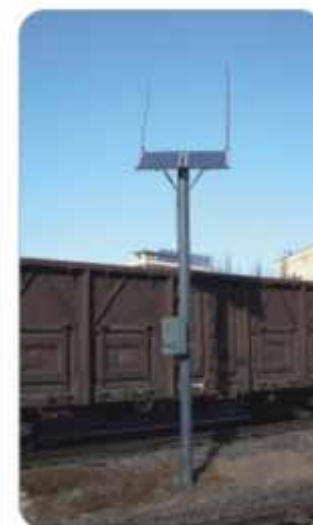
铁路监控设备供电系统 Railway Monitoring Equipment in PV stand-alone System
