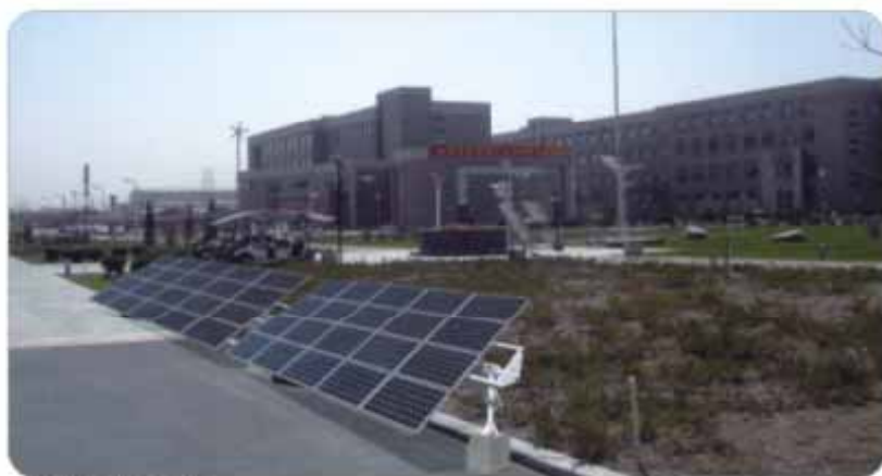
沈阳工程学校并网发电系统 Grid electrical power system in Shenyang Institute of Engineering
