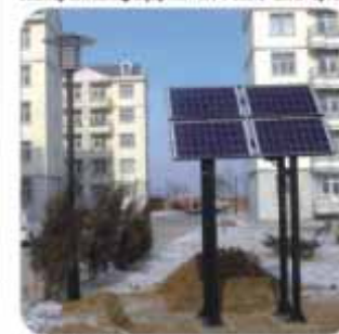
庭院灯供电系统 Garden Light in PV stand-alone System
