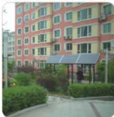
沙岭小区庭院灯供电系统 Shaling Community Garden Light PV Power Supply System
